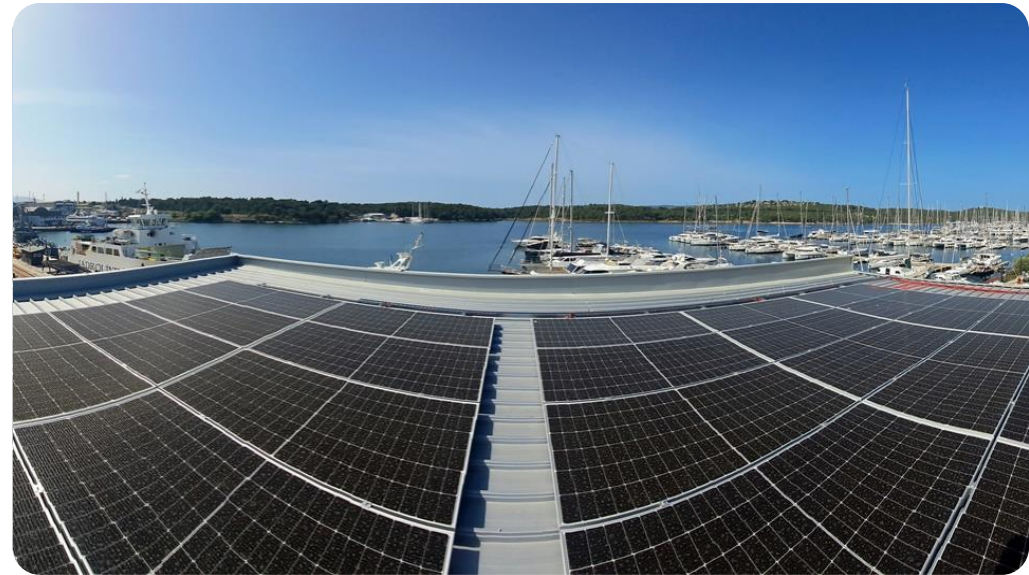
Šibenik: Iskra Shipyard Solar power plant
