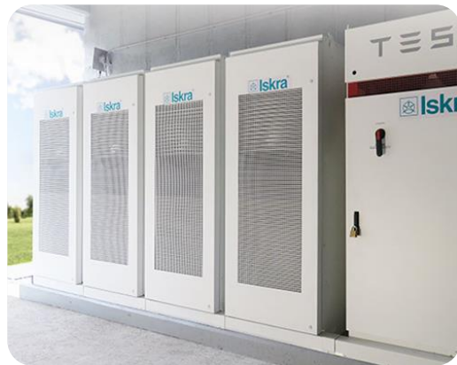
Kranj: Battery storage system
